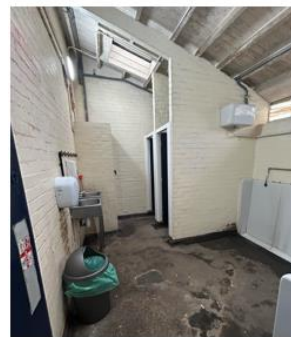
Figure 78. Poor quality existing WCs at the Station car park.
