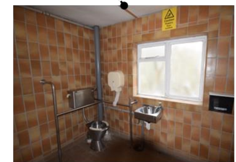
Figure 76. Accessible Public WC Grosmont.
