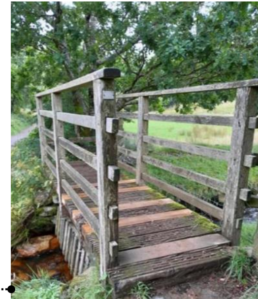
Figure 36. Bridge to be made good under current work schedule. Image © Lake District National Park Authority.
