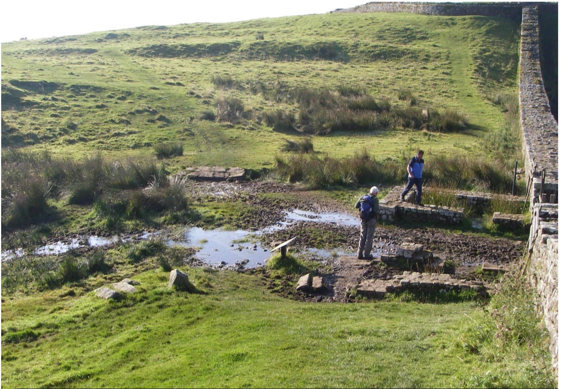
Drainage problem: Visitors are forced to walk on top of the monument
